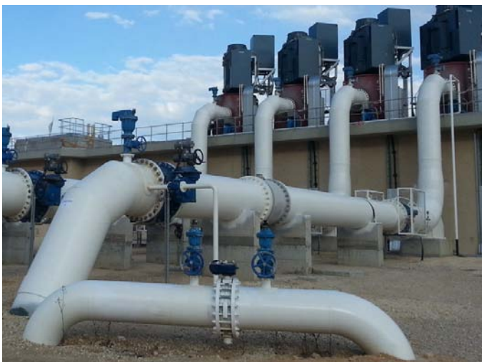
Water pump station
